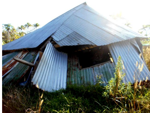
house at Tuvana-I-Ra damaged by cyclone 2018
